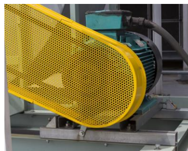
Fig 19A: Fixed guard on rotating shaft/coupling
